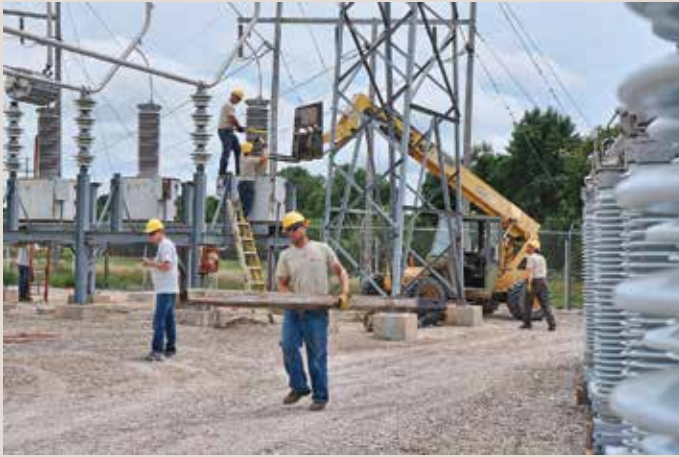
Corn Belt Power Cooperative, wholesale power supplier for your cooperative, recently upgraded its Hope Switching Station near Humboldt. The upgrade improves system reliability and provides backup should future line trips occur.
